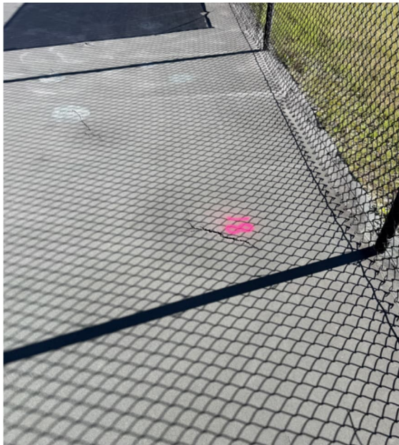
Photo 3: Small cracking at DCP-18
