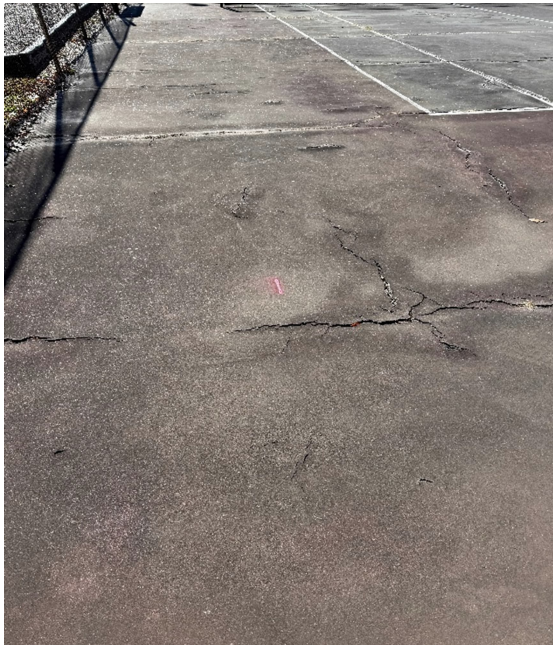
Photo 1: Cracking, depressions, and water stains at DCP-1
